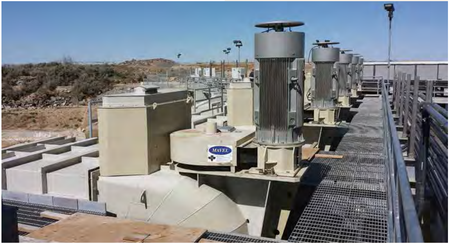
The installed Mavel generators up close.
